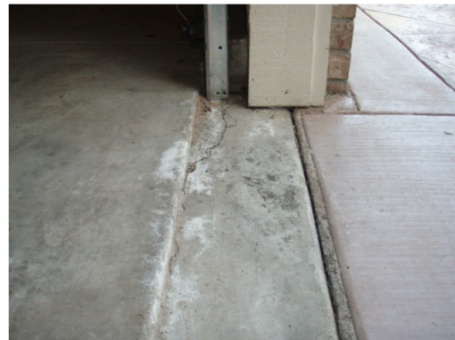
Built in depressions in the garage floor will help keep water out of the garage.
