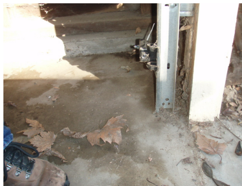
Light sensor too high off the floor is a child safety hazard
