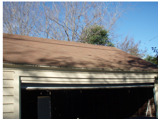
Sagging header on older garage
