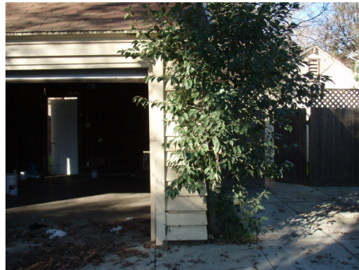
Leaning wall on detached garage
