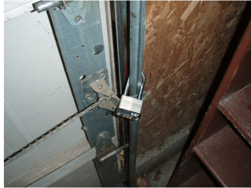
A pad lock in the garage door track can cause the door to fall off the tracks
