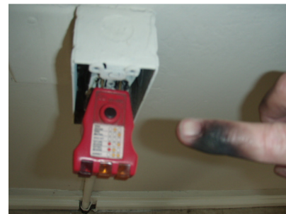
This outlet was defective and exploded. The tester was undamaged
