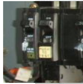
GFCI circuit breakers can also be installed inside electrical panels
